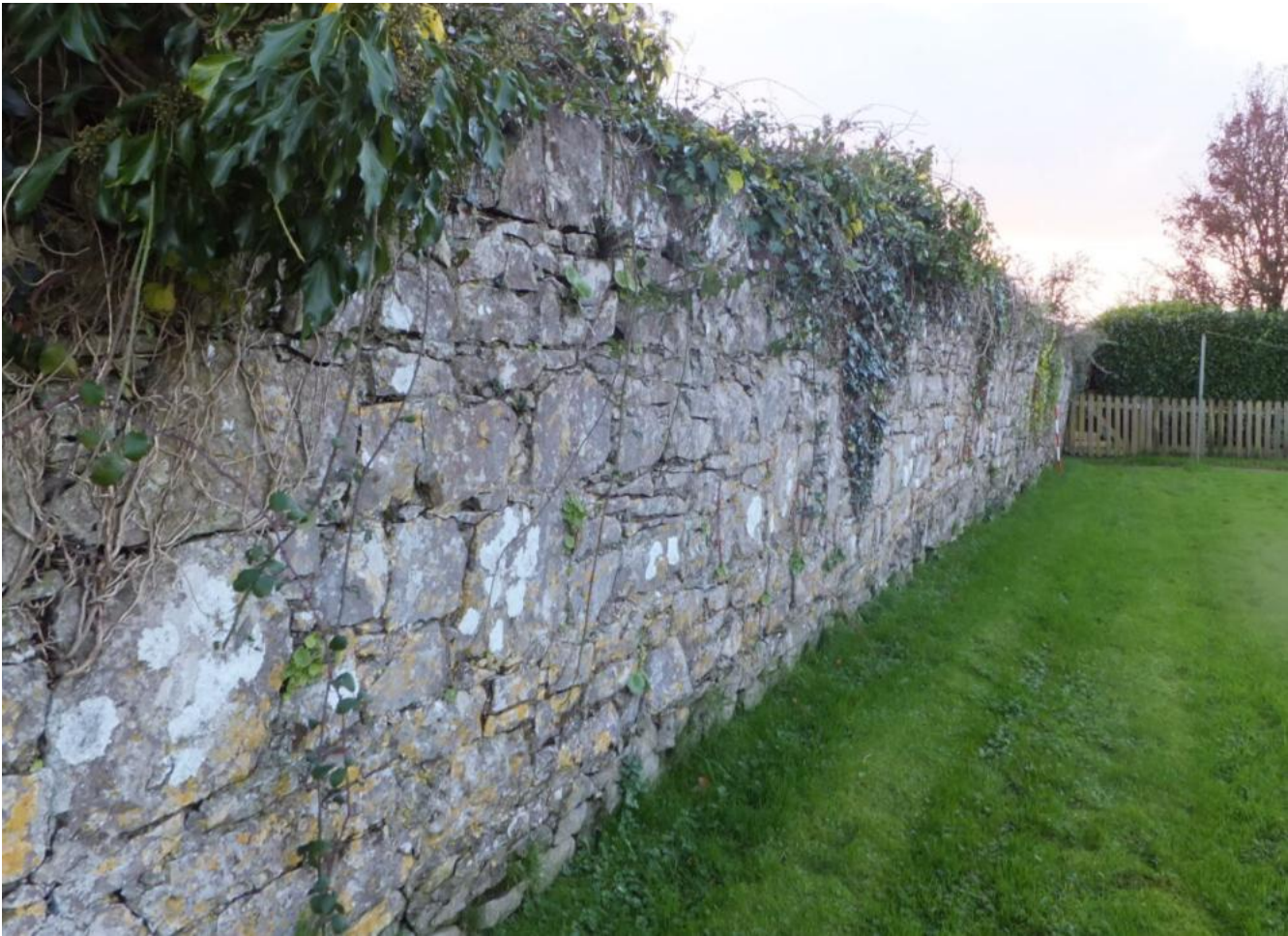
Long view of outer face of wall, prior to collapse; from east
