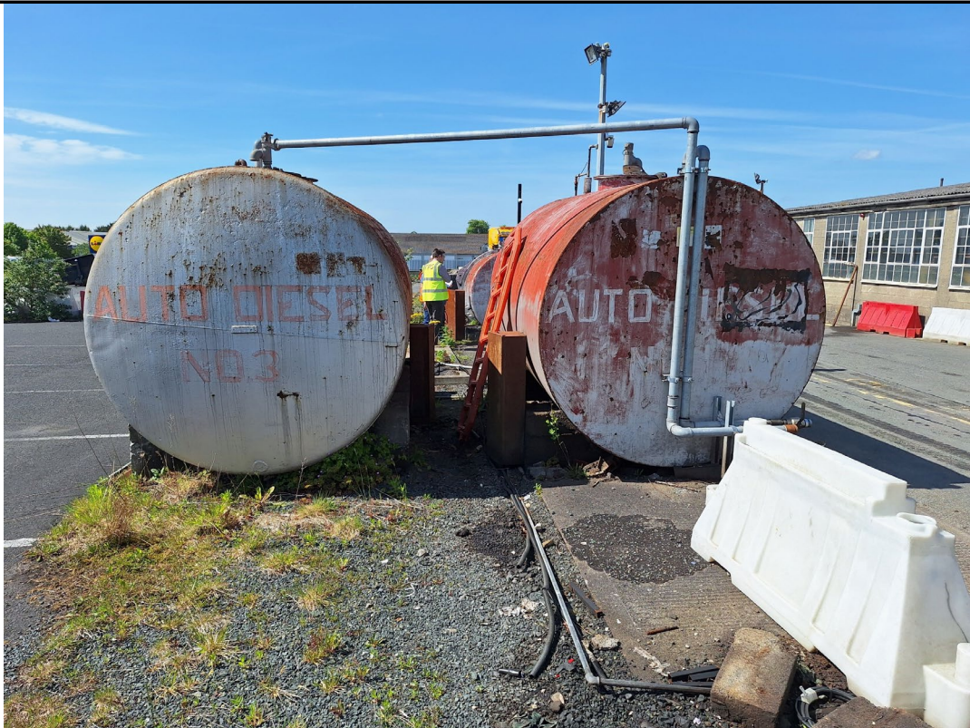
Image 11: View of 2 No. diesel AST (5,000-litre approx) south of workshop building, facing west. Tanks of steel construction, un-bunded, un-protected, ground staining evident.
