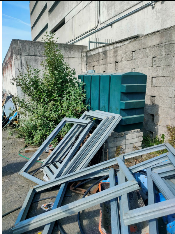
Image 15: View of 1 No. 1,200-litre approx. AST (heating oil) located in Water Dept exterior yard, northern site boundary, facing northwest. Un-banded, on concrete block base.
