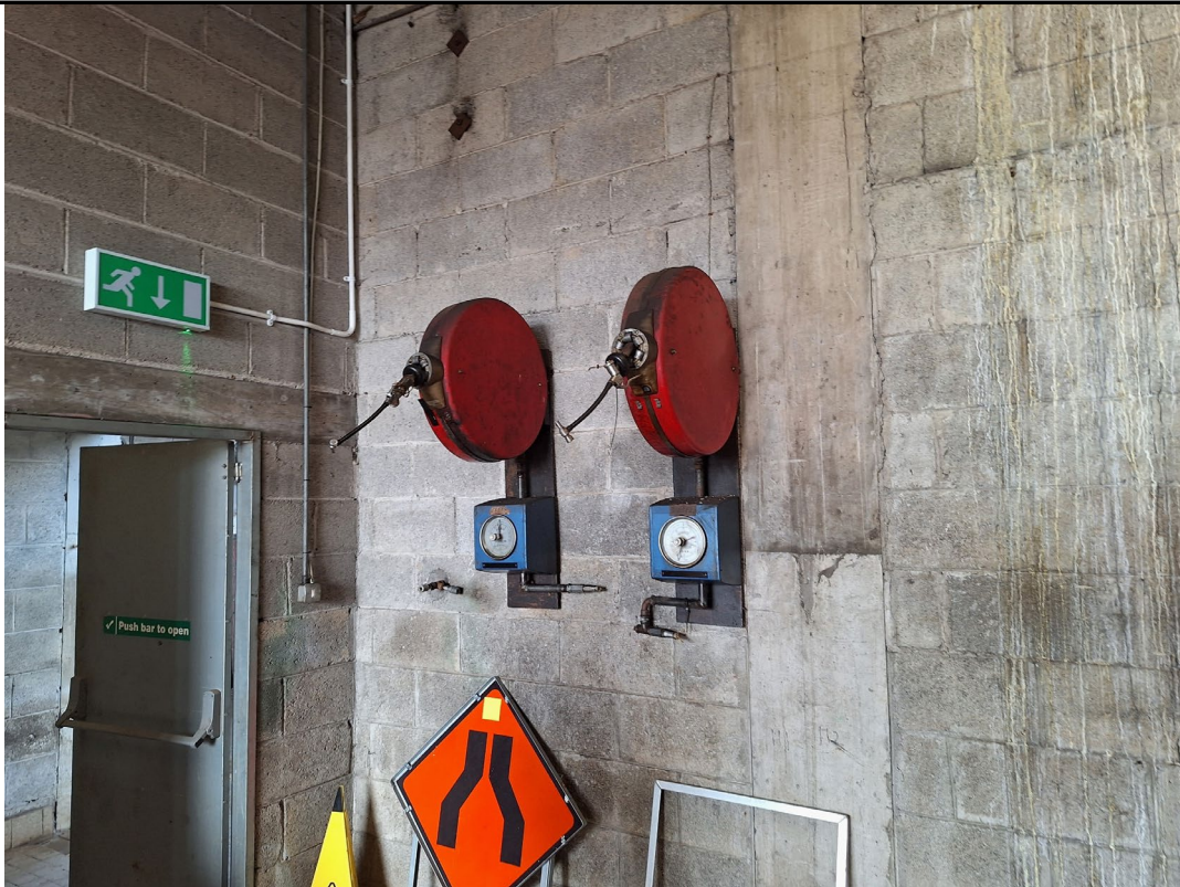
Image 29: View of interior wall mounted oil / fuel dispensers and gauges located on east side of workshop.
