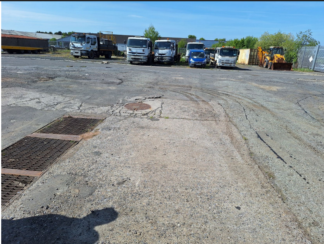
Image 17: View of northwest of site, facing southwest. Catch-pit visible on left in former wash-down area. Broken concrete and asphalt ground surface typical of site exterior.
