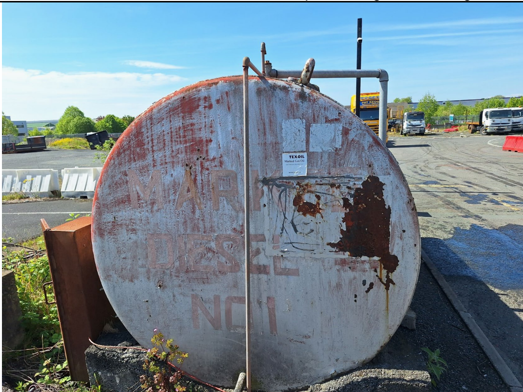
Image 12: View of green diesel AST (5,000-litre approx.) located south of workshop, facing west. Concrete plinth visible at base, un-bunded, ground staining observed.
