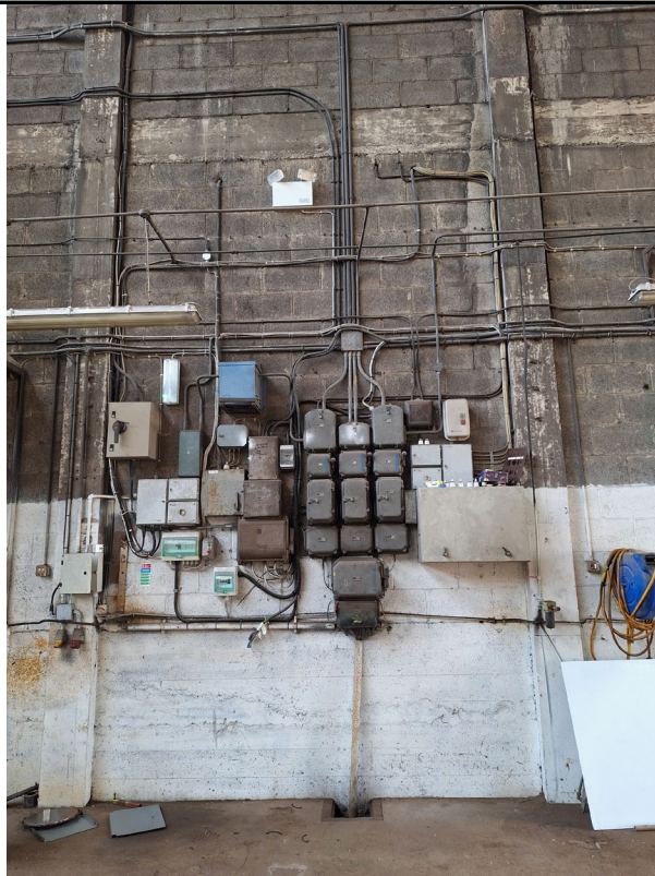
Image 25: View of electrical fuse boxes and circuit breaker panels on south interior wall of workshop building.
