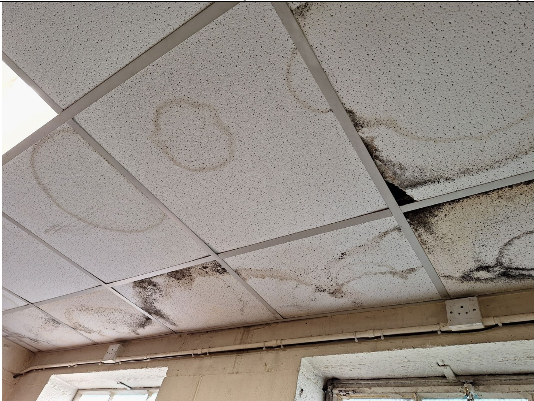
Image 32: View of ceiling in workshop kitchen / canteen, with water damage and mold visible on drop ceiling tiles and painted block walls.
