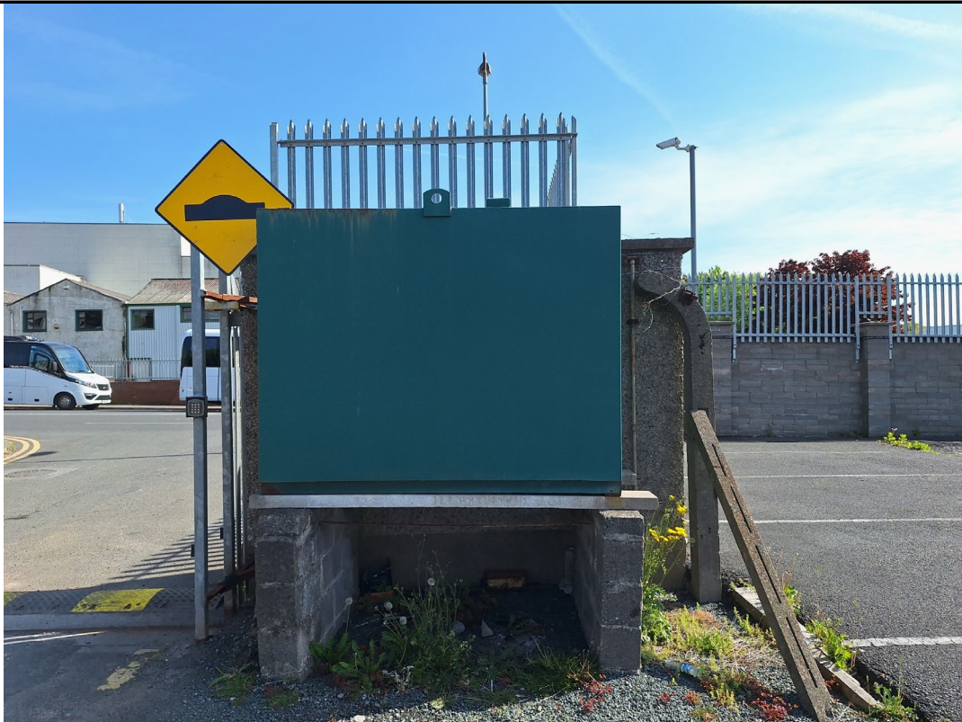
Image 9: View of heating oil aboveground storage tank (AST) adjacent to main site entrance gate, approx. 1,200-litre volume, steel construction.
