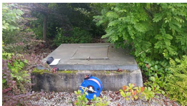
Photo 3. BH 2 pump chamber
