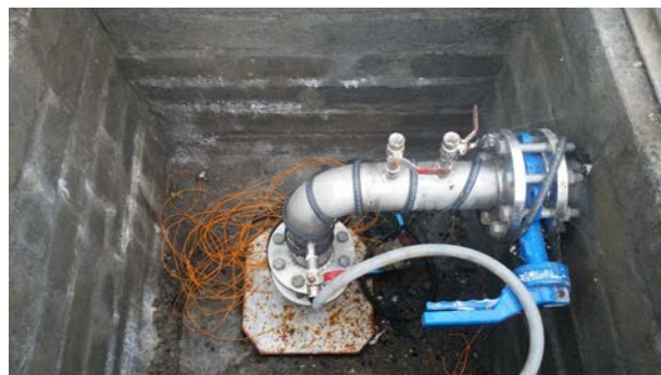
Photo 2. BH 1 headworks in pump chamber
