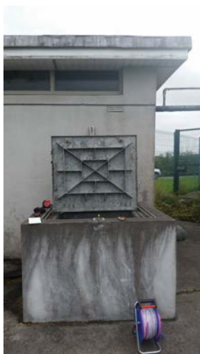
Photo 1. BH 1 pump chamber
