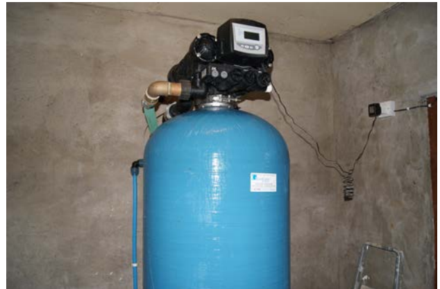
Photo 3 – Iron and manganese filtration unit
