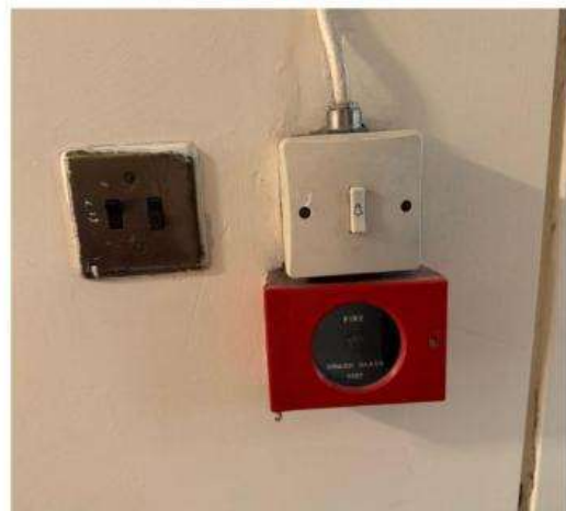
SWITCHES / MANUAL FIRE CALL POINT
