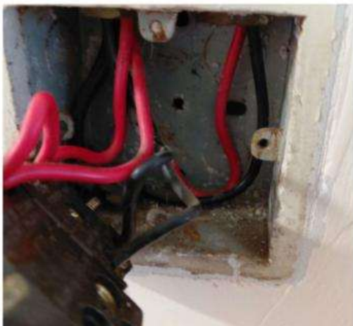
OLD RED & BLACK CABLING
