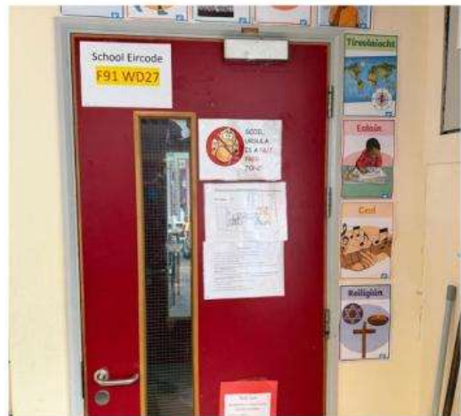
NO EMERGENCY LIGHTING
