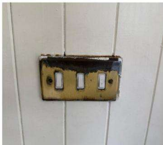
OVERHEATED SWITCH PLATE
