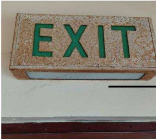
OBSOLETE EML FITTING
