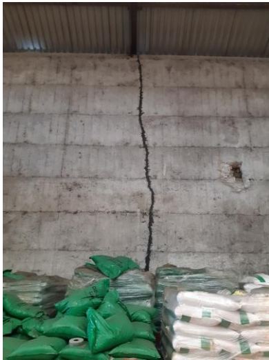
Evidence of vertical stress cracks within the building structure.
