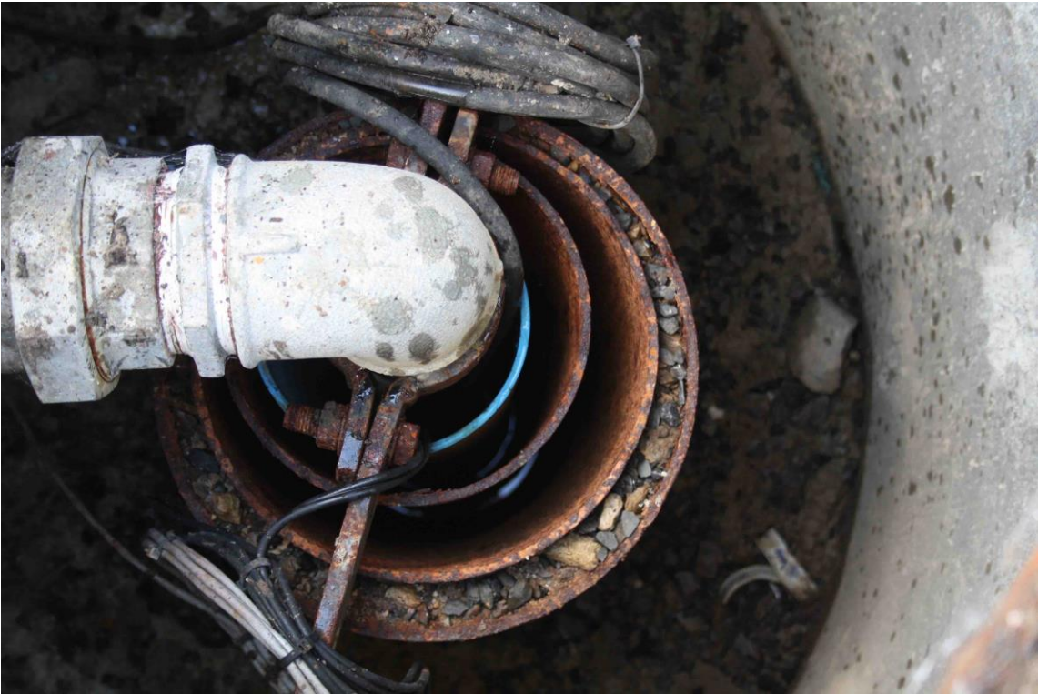
Photo 2 PW1 Wellhead arrangement
