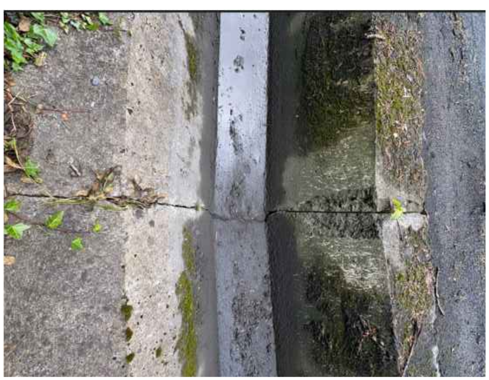
EXAMPLE OF EXISTING CRACK
