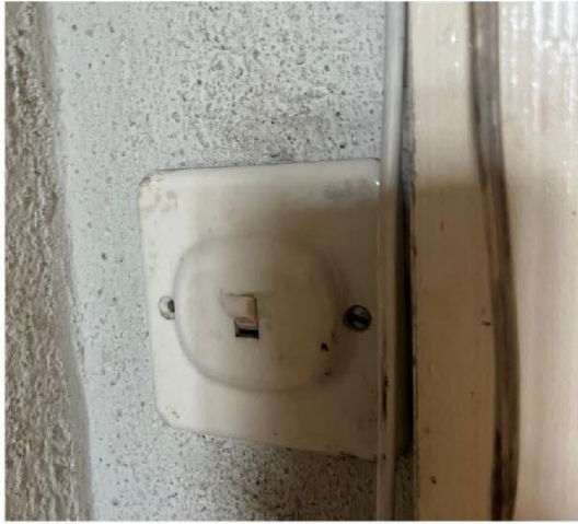
OBSOLETE ROCKER SWITCH
