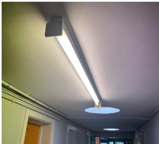
CORRIDOR - DEFECTIVE FLUORESCENT LIGHTING
