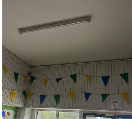
OBSOLETE CLASSROOM FLUORESCENT LIGHTING
