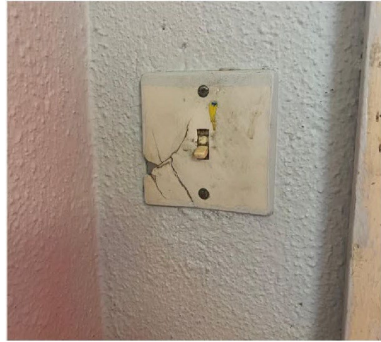
CRACKED AND DAMAGED ROCKER SWITCH
