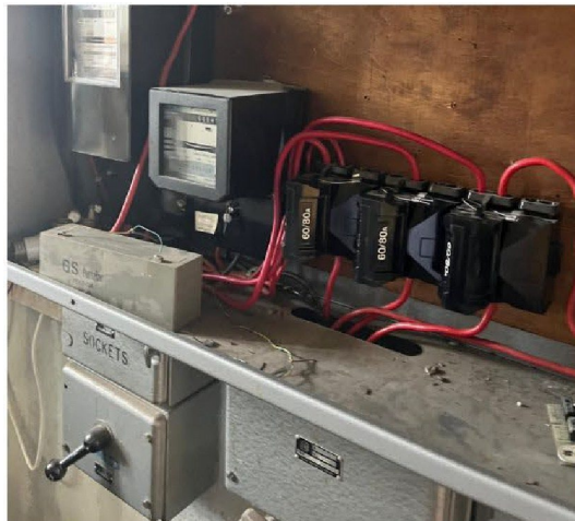
EXPOSED WIRING AND FUSE CARRIERS
