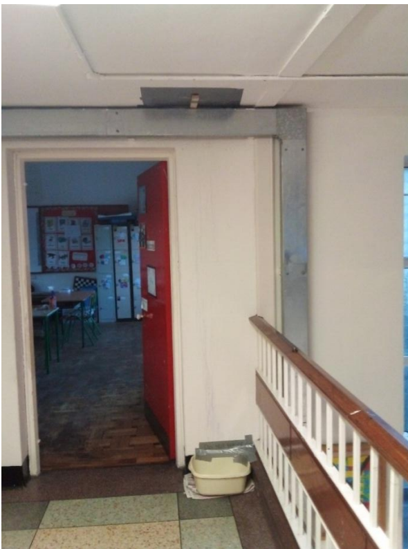
Figure 3: Evidence of destructive impact of the flat roof failure inside the school building. Active water ingress entering a main corridor right outside a classroom door and stairwell landing.
