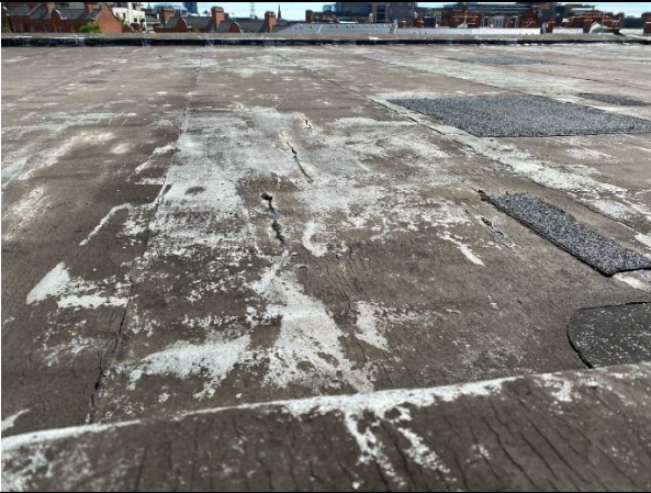
Figure 2: Existing roofing felt – evidence of blistering and surface pitting, thermal cracking, and advanced UV degradation across the roof deck. Torch-on felt patches have assisted in slowing down the failure but has not prevented additional water ingress. Repairs are no longer working. The surrounding asphalt/felt substrate is too degraded, brittle, and porous to hold a watertight seal.
