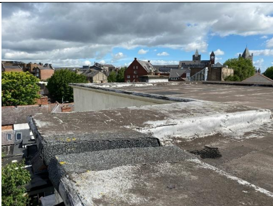
Figure 1: Overview of area of roof in need of work including chimney, note the patch repairs at the outlet
