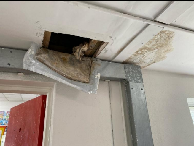
Figure 4: rainwater from the leaking roof has saturated the ceiling fabric. The sagging and deep staining indicate that this section of the ceiling is being damaged by water ingress. The active leak tracks directly alongside the main galvanized electrical/services trunking, increasing health & safety, and fire hazard risks for occupants.
