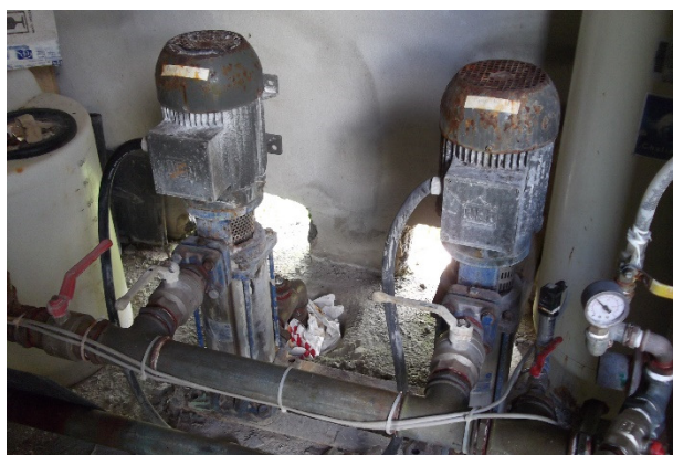
Photo 6: Pumps and holes in pump house wall beside open pump sump
