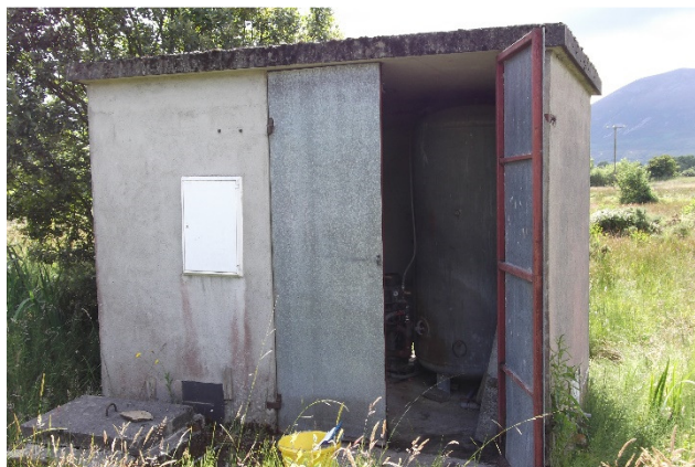
Photo 4: Pump house over sump
