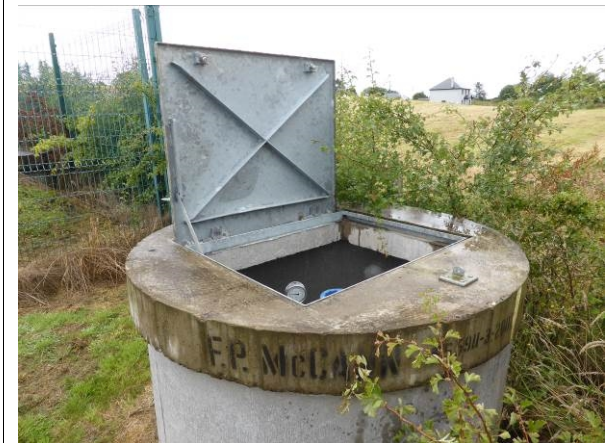
Photo 5: Current Source Borehole chamber access
