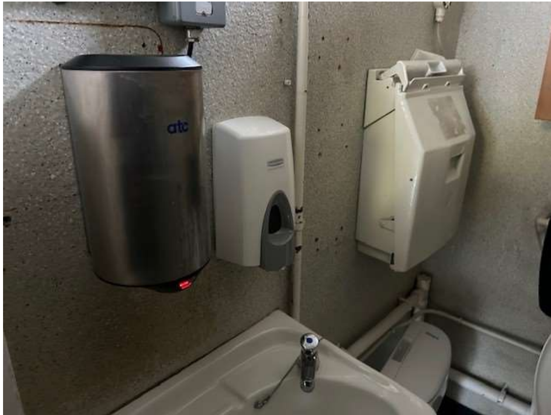
Interior view of existing WC with duct, WHB and toilet roll holder compromising the usable width.
