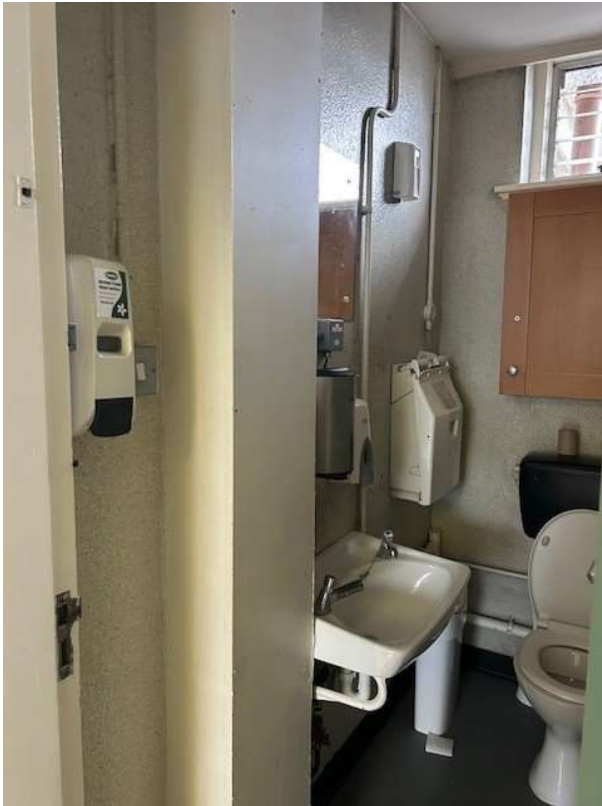
Interior view of existing WC with duct, WHB and toilet roll holder compromising the usable width.
