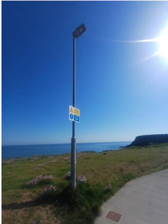
Typical street light (single lamp)
