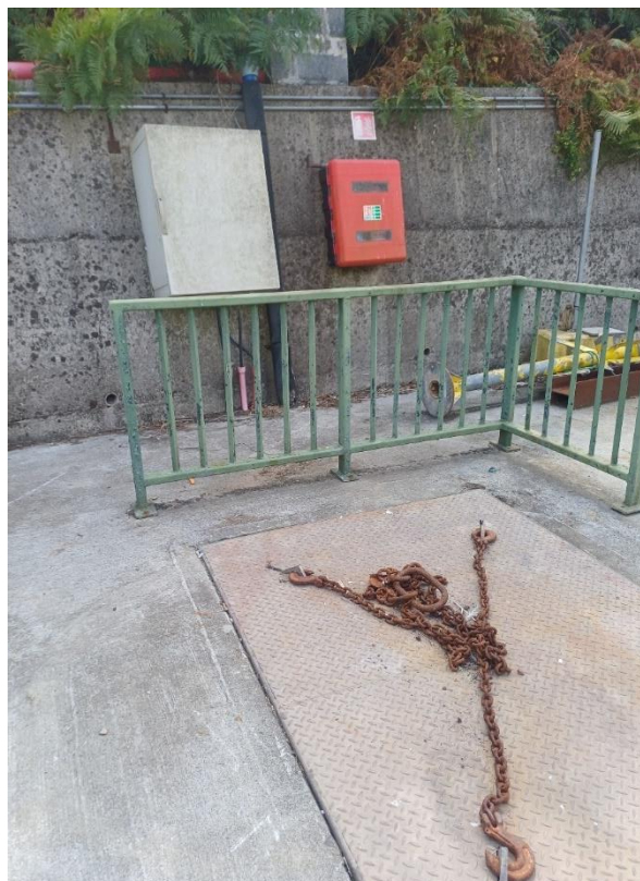
Septic Tank / Pump
