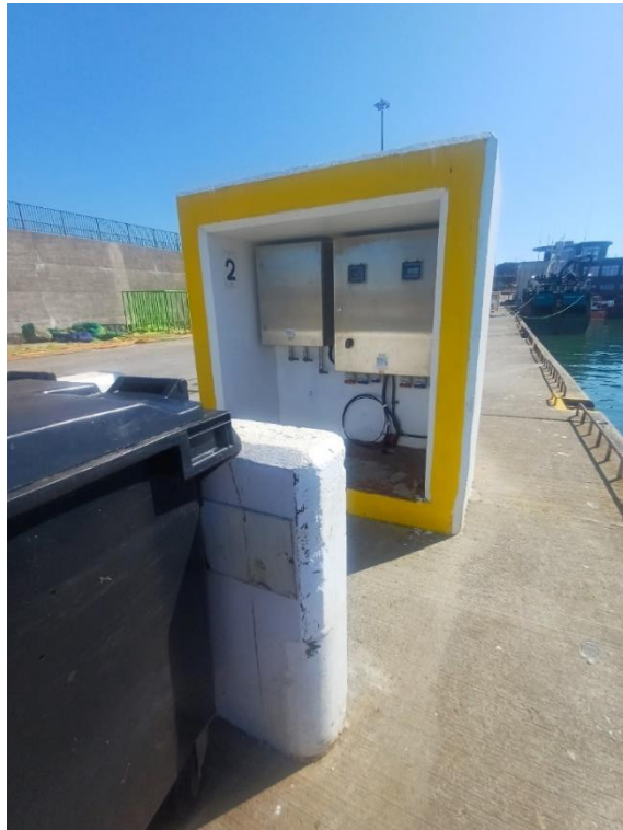
Typical Power Box
