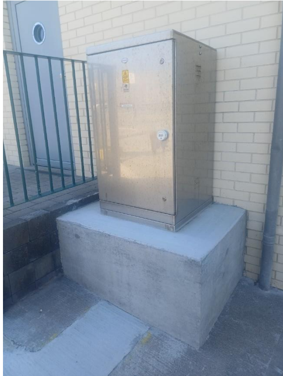
Weighbridge Control Panel
