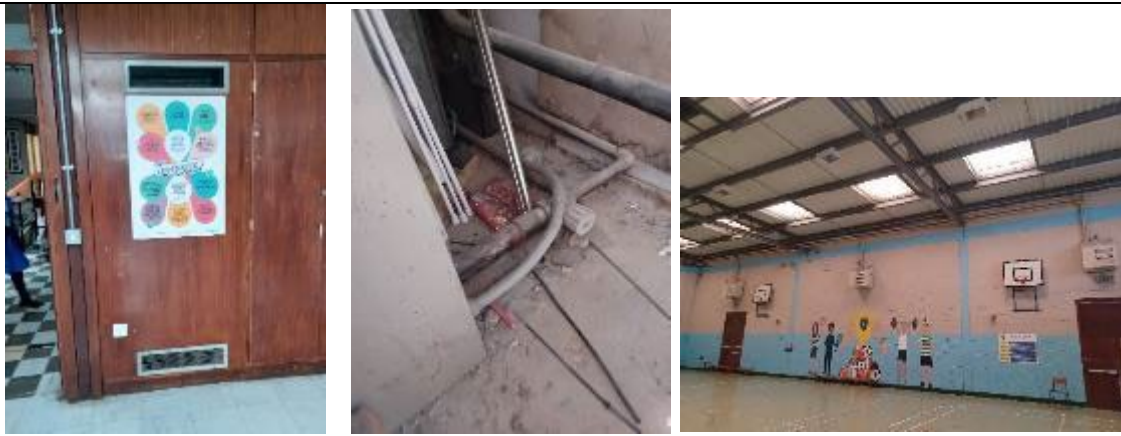
Figure 3/3a/3b -Fan assisted convectors / Sports Hall unit heaters at high level
