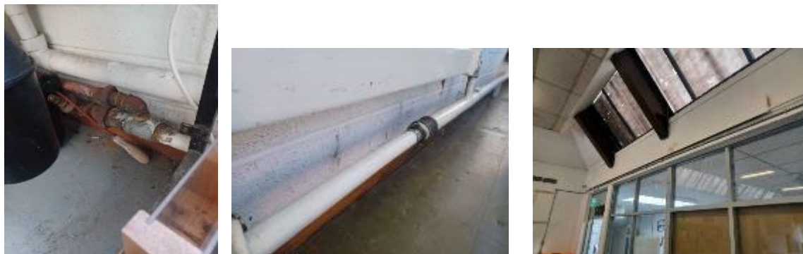
Figure 2/2a/2b - Corrosion of Classroom heating pipework / Evidence of pipework repairs to heating pipework / Radiators at high level in Assembly Hall
