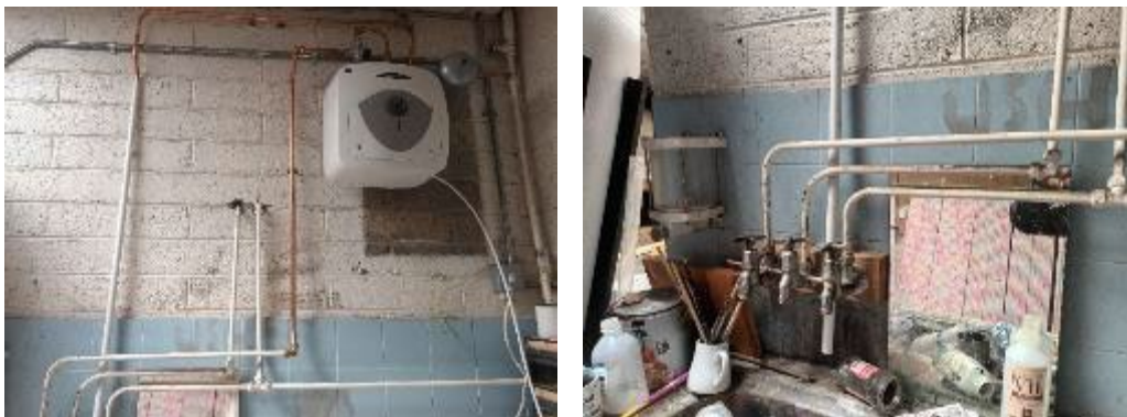
Figure 4/4a - Hot & cold-water services pipework in poor condition
