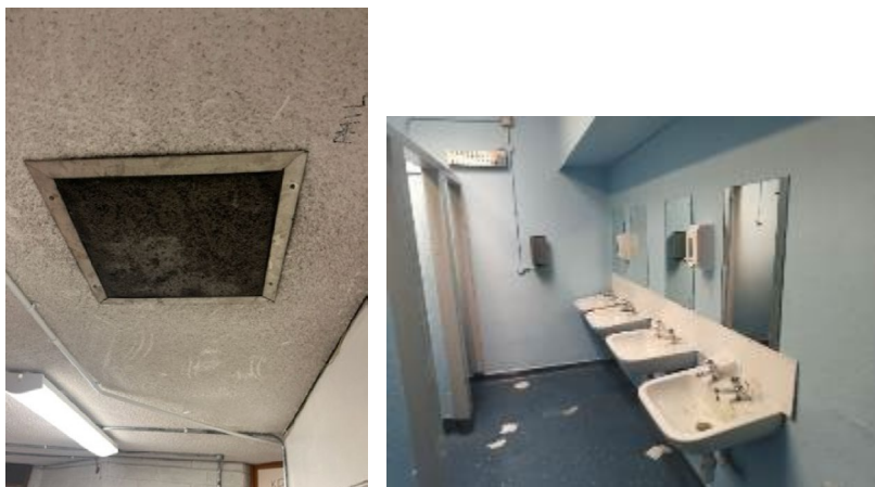
Figure 5/5a -Typical extract ventilation grille in Assembly Hall in poor condition/Internal Toilets with no mechanical ventilation
