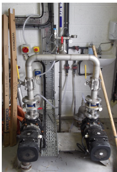
Photo 6: Raw water duty and stand-by pumps
