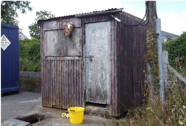
Photo 1: Local Authority sump, external access and treatment shed
