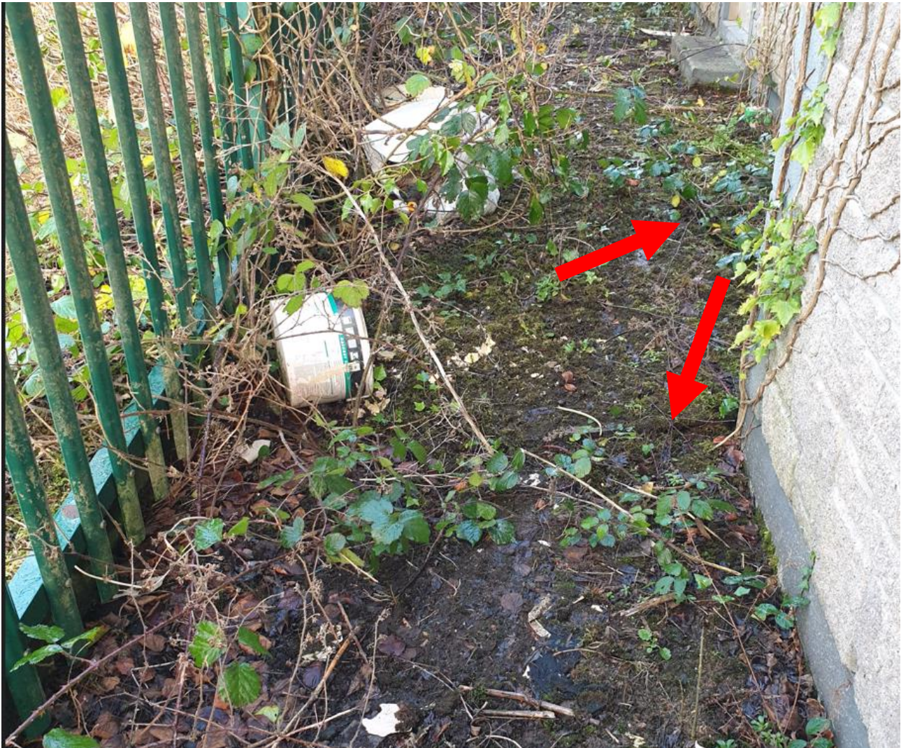
Photograph 13 Footpath to front of northern elevation of 'Block B' building (to be demolished) – Note location of significant cracking (masked by overgrowth).
