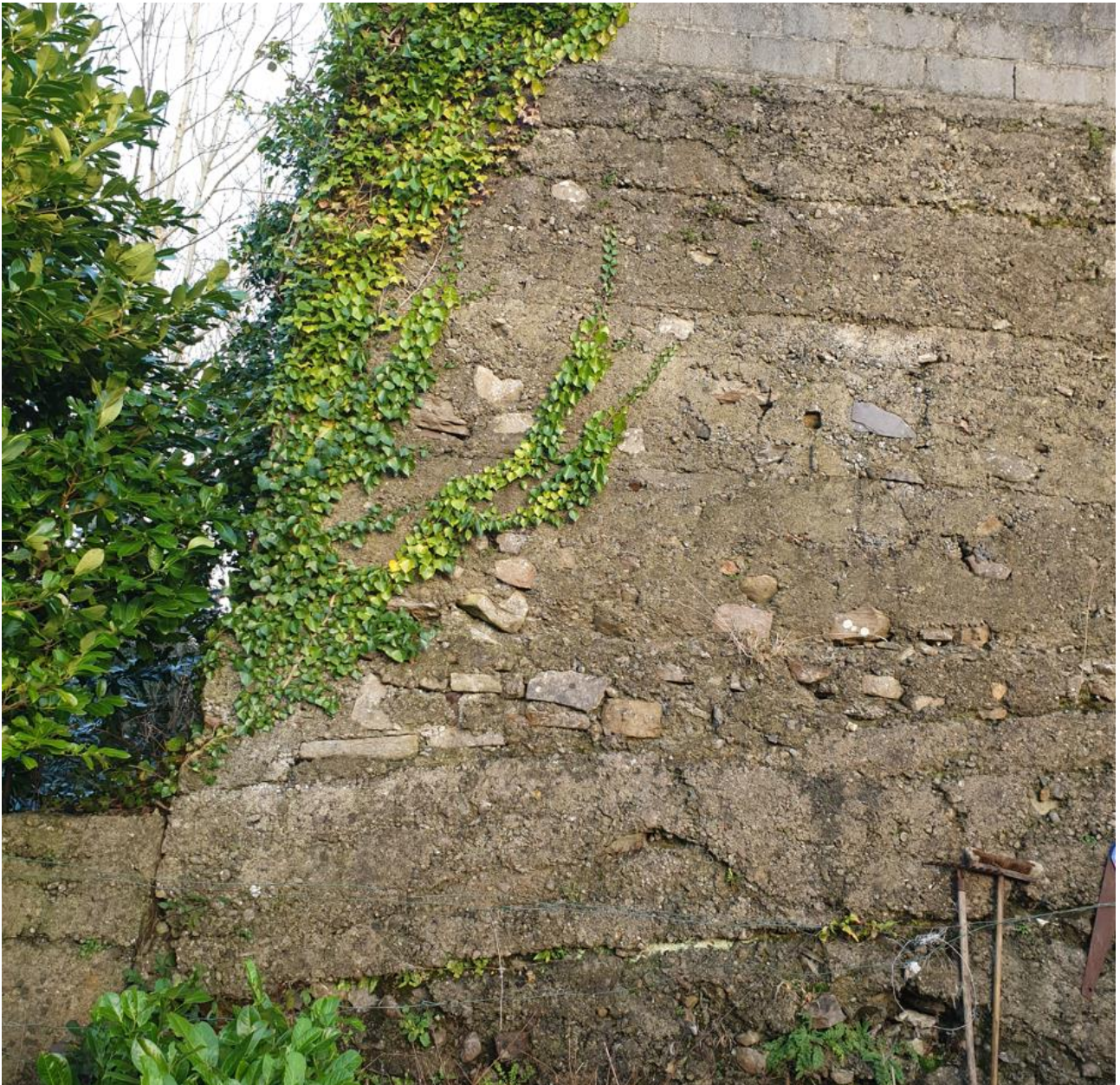
Photograph 5 West face (northern end of structure). Note general condition, including construction joint cracking.
