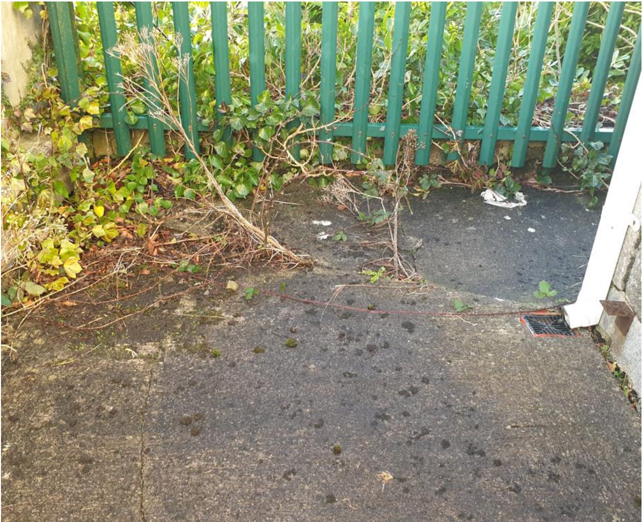
Photograph 14 Footpath to northwestern corner of 'Block B' building (to be demolished) – Note significant cracking (masked by overgrowth).
