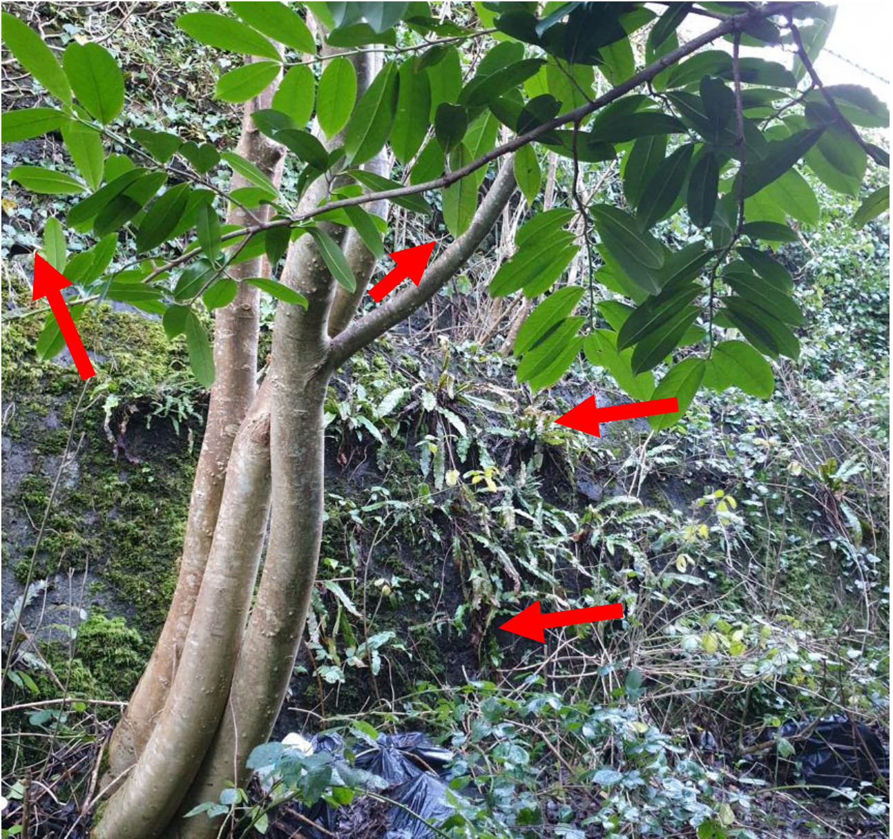
Photograph 8 Northern face of structure – Note generally condition of structure including proximity of trees and root infiltration / penetration. Location of significant cracking indicated (masked by overgrowth).
