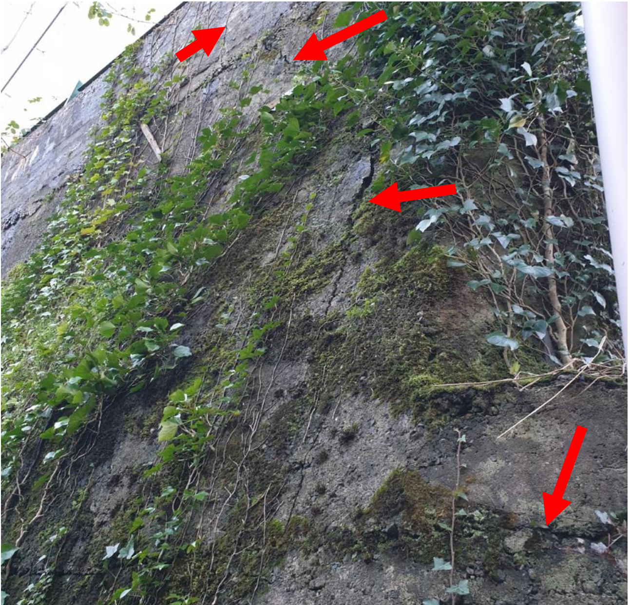
Photograph 9 Eastern face of structure – Note generally condition of structure including root infiltration / penetration. Location of significant cracking indicated.
