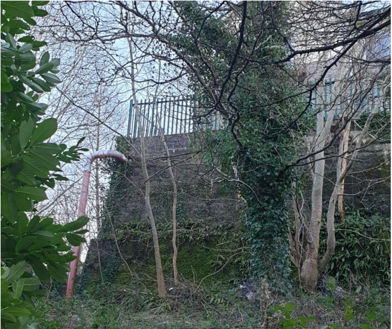
Photograph 6 Northern face of structure – Note generally condition of structure including proximity of trees and root infiltration / penetration.
