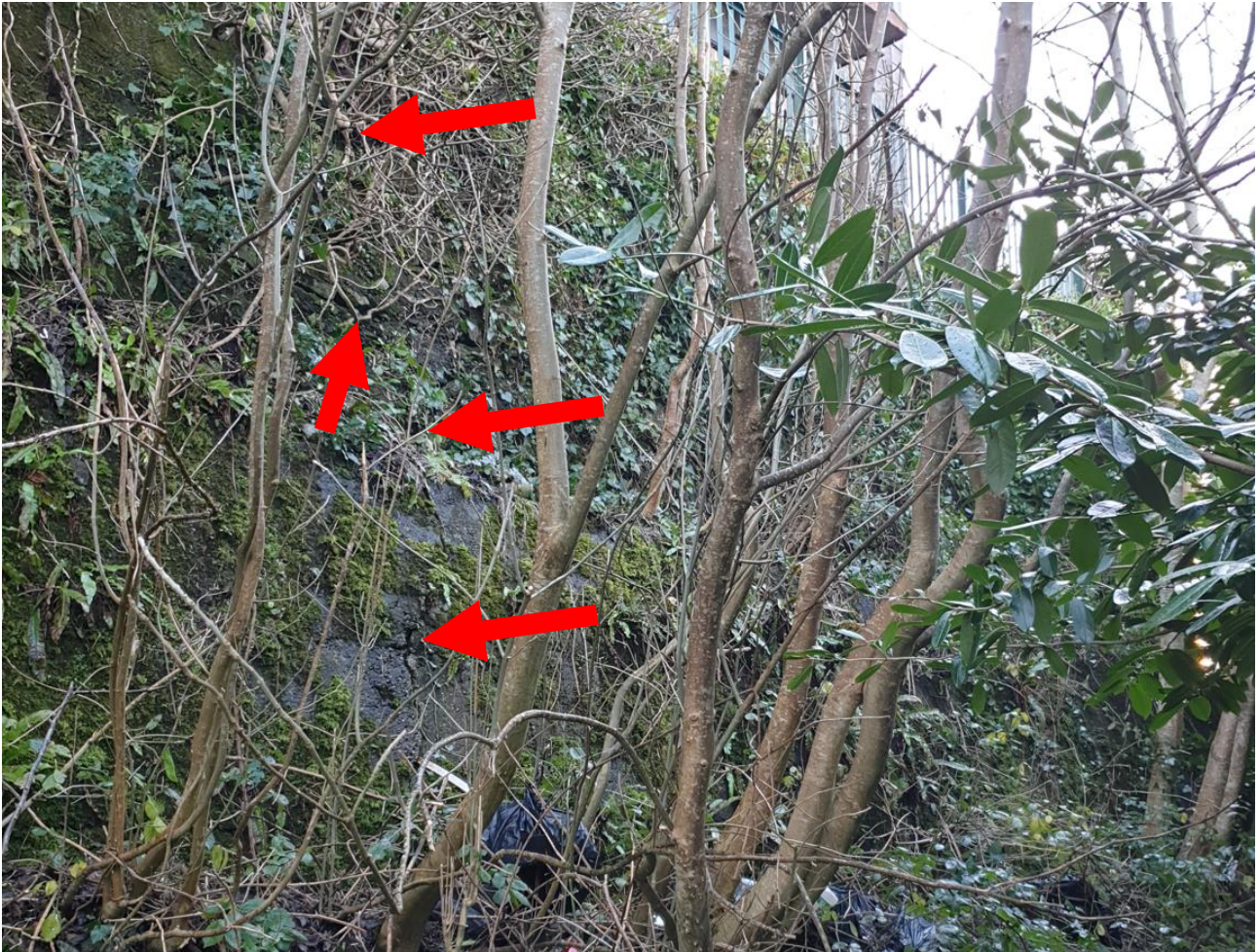
Photograph 7 Northern face of structure – Note generally condition of structure including proximity of trees and root infiltration / penetration. Location of significant cracking indicated (masked by overgrowth).
