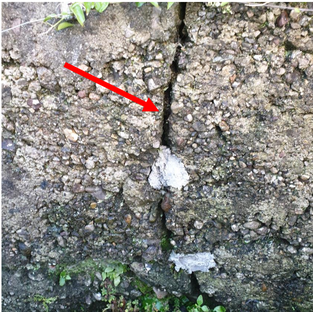
Photograph 3 West Face of structure. Note cracking to base of wall.
