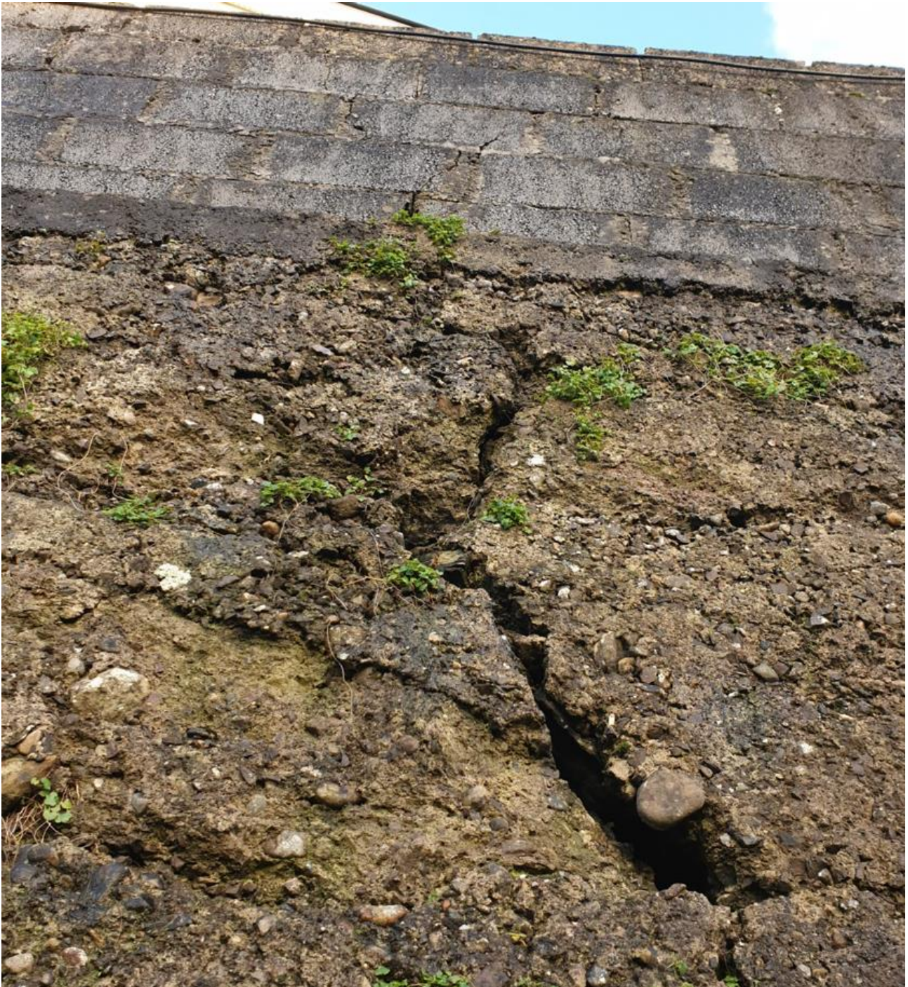
Photograph 4 West face of structure. Note significant cracking to original wall and to block wall above.
