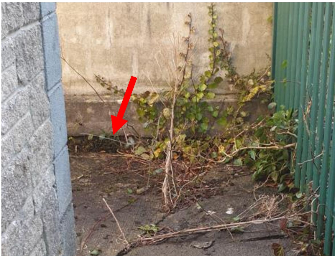
Photograph 15 Footpath to northwestern corner of 'Block B' building (to be demolished) – Note exposed wall, indicating significant drop in footpaths.
