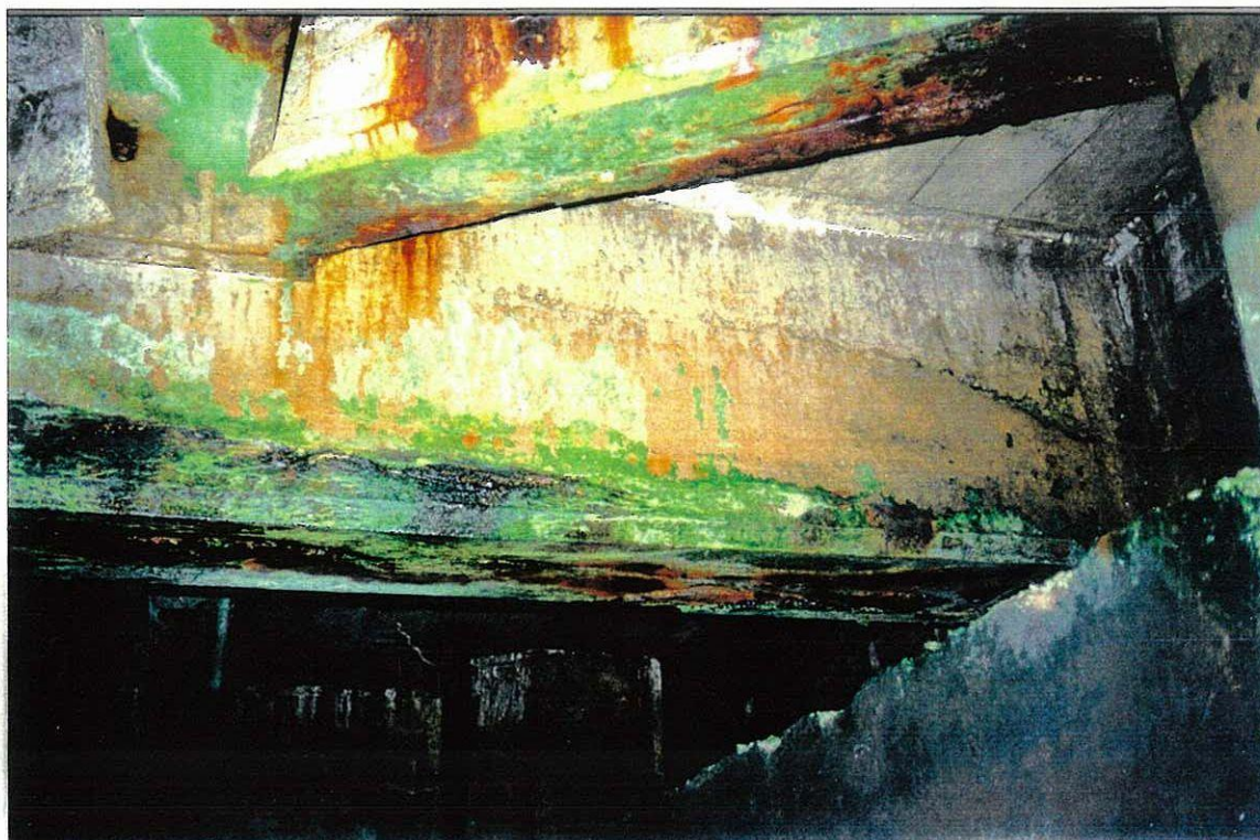
P.7. - DETERIORATION OF BEAM ELEMENTS
