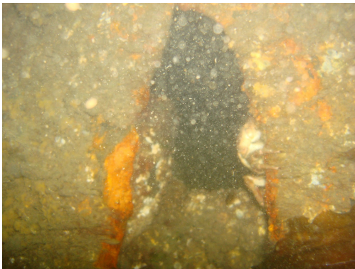
Plate 5 – Hole in sheet pile wall at CH15m
