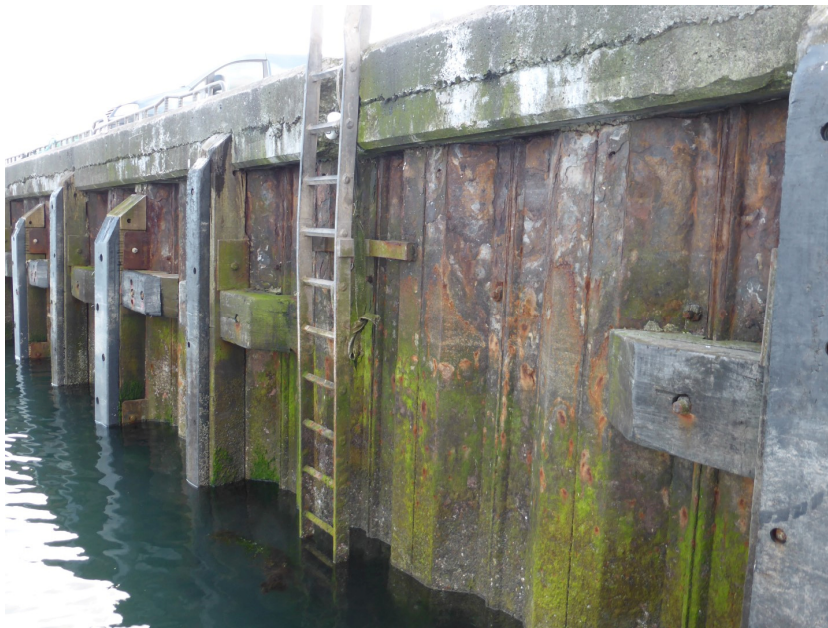
Plate 4 – Corrosion of sheet piles in Splash zone
