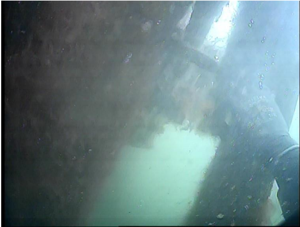
Photograph 23: Defect to fender at Ch 163
