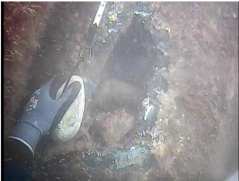
Photograph 12: Void at Ch 187
