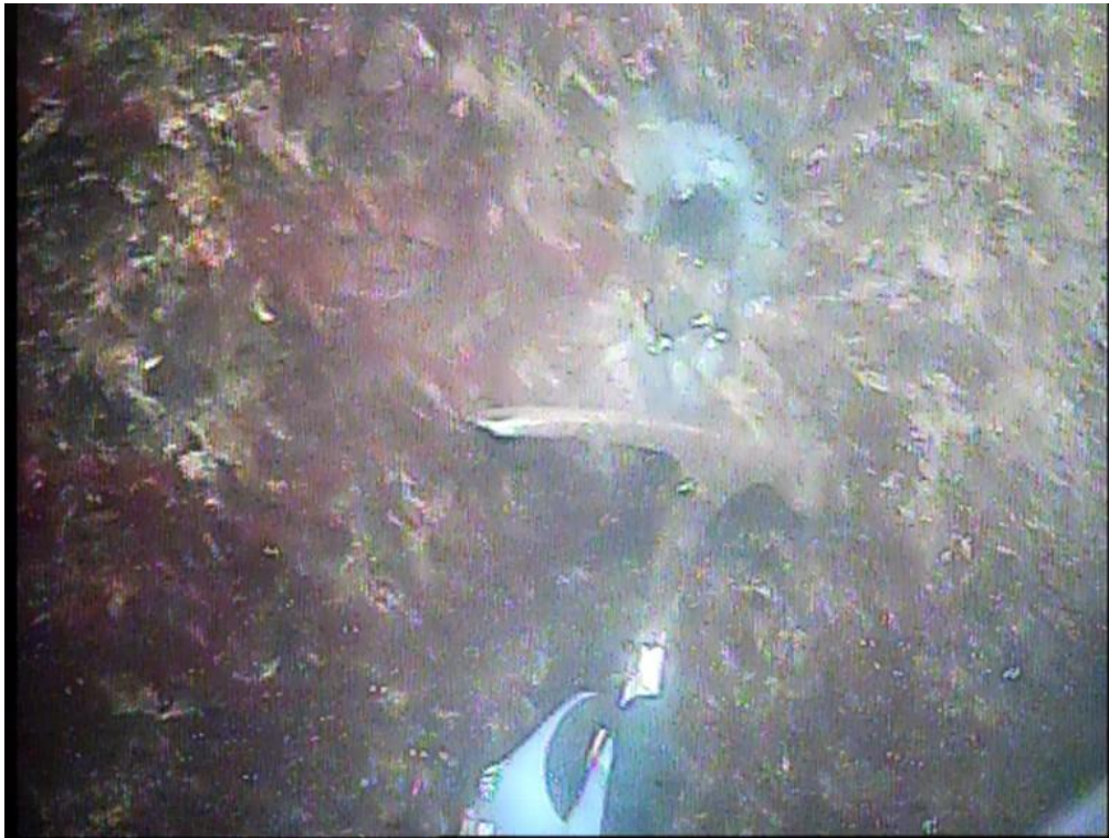
Photograph 13: Void at Ch 190
