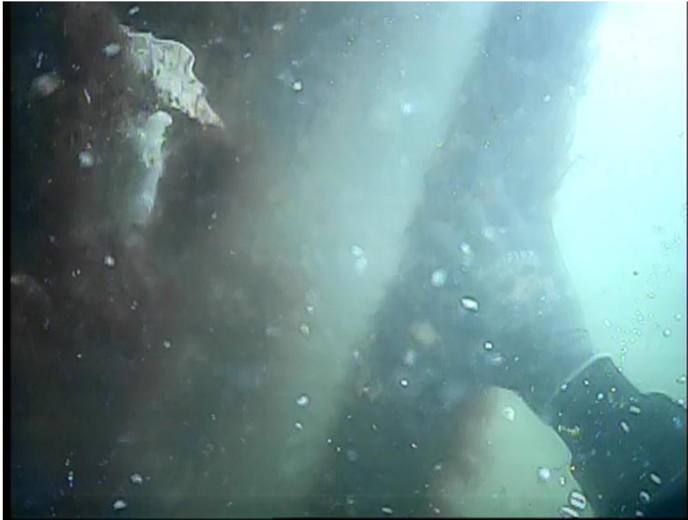
Photograph 21: Defect to fender at Ch 148
