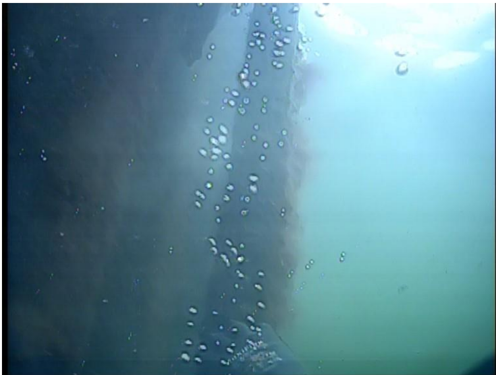
Photograph 18: Defect to fender at Ch 129
