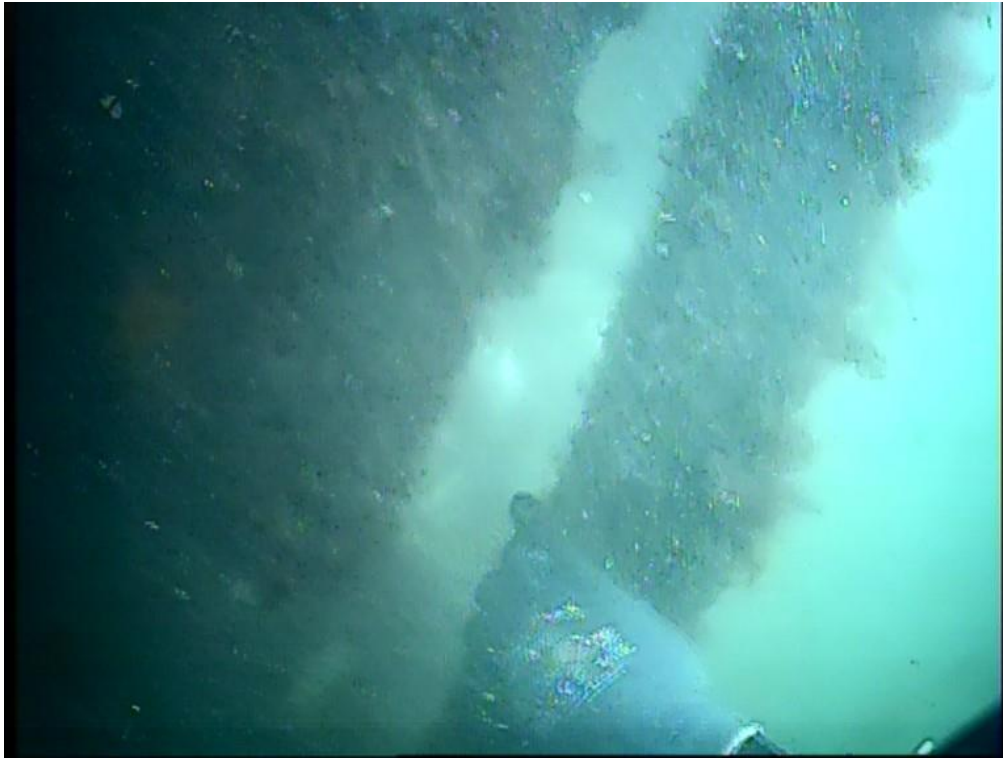
Photograph 19: Defect to fender at Ch 133
