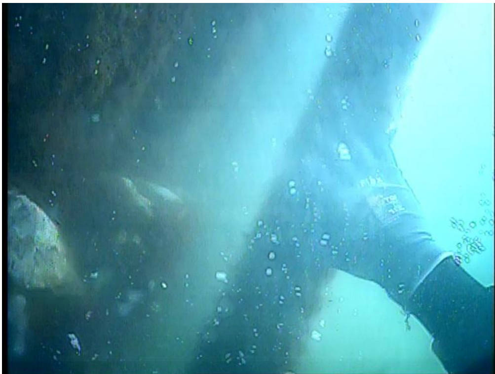
Photograph 20: Defect to fender at Ch 141
