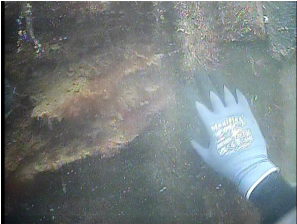
Photograph 24: Defect to the fender cross member at Ch 167
