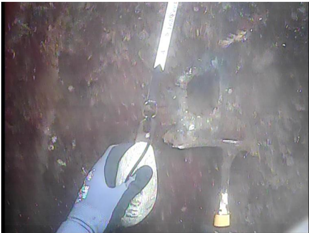
Photograph 14: Void at Ch 198
