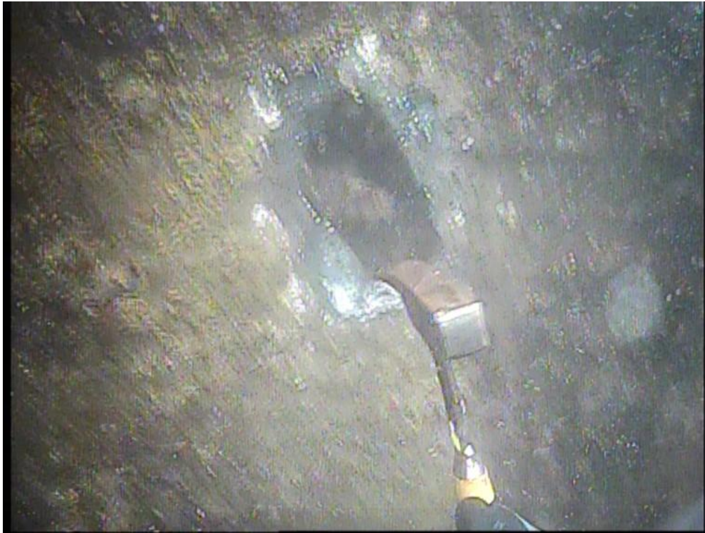
Photograph 11: Void at Ch 178
