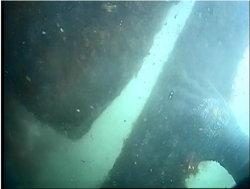
Photograph 17: Defect to fender at Ch 125
