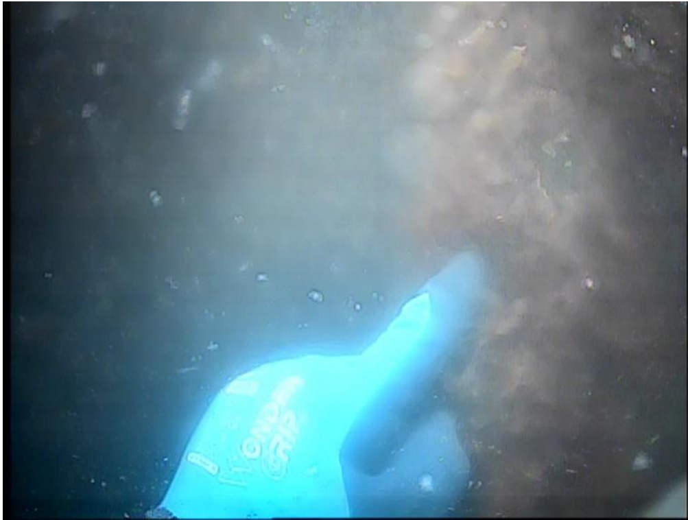
Photograph 15: Defect to fender at Ch 87
