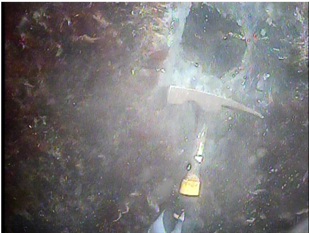
Photograph 10: Void at Ch 67
