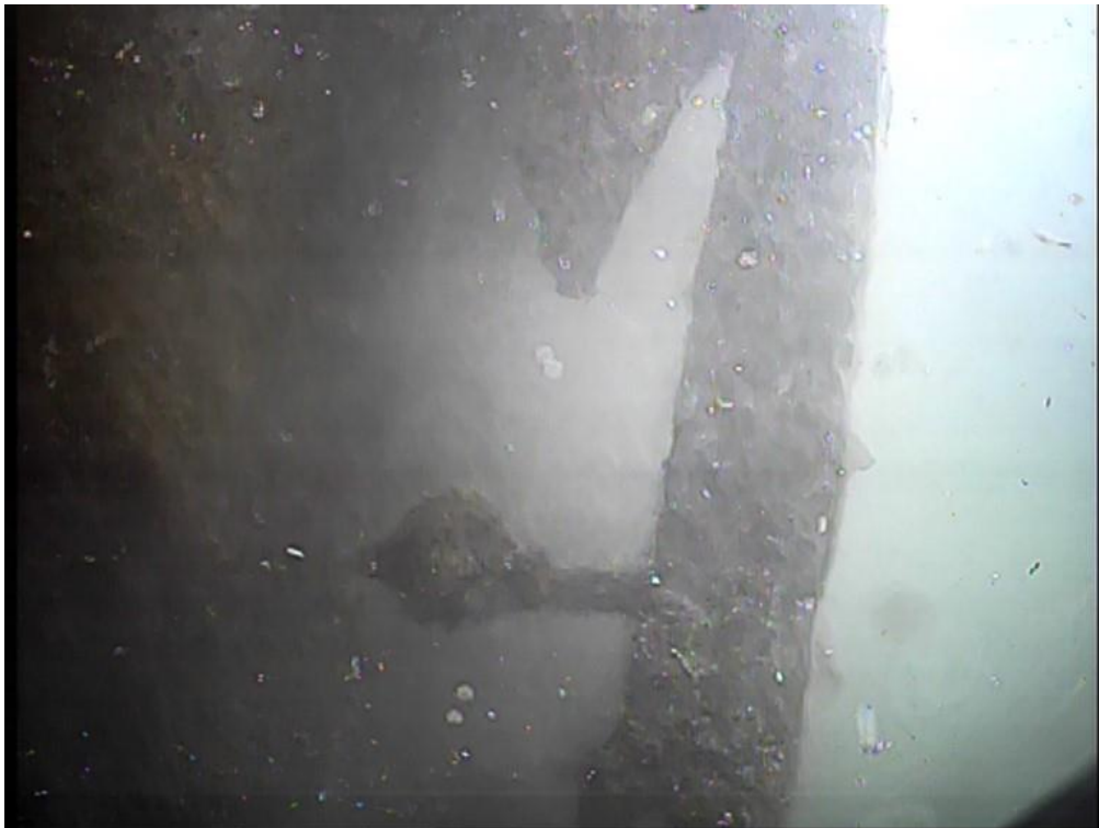
Photograph 16: Defect to fender at Ch 106
