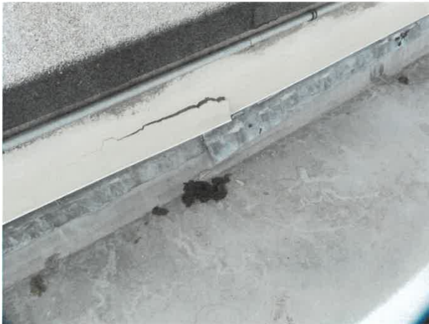
View of faulty flashing detail
