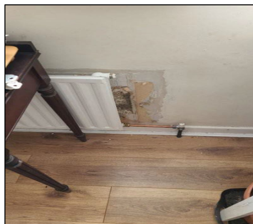
Figure 31: Unsightly patches pipework
