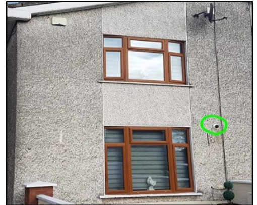
Figure 13: Adequate evidence supplied by flue
